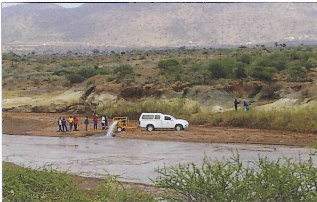
Cleaning of pump chambers in the Moutse River for the Motoulela Village.
