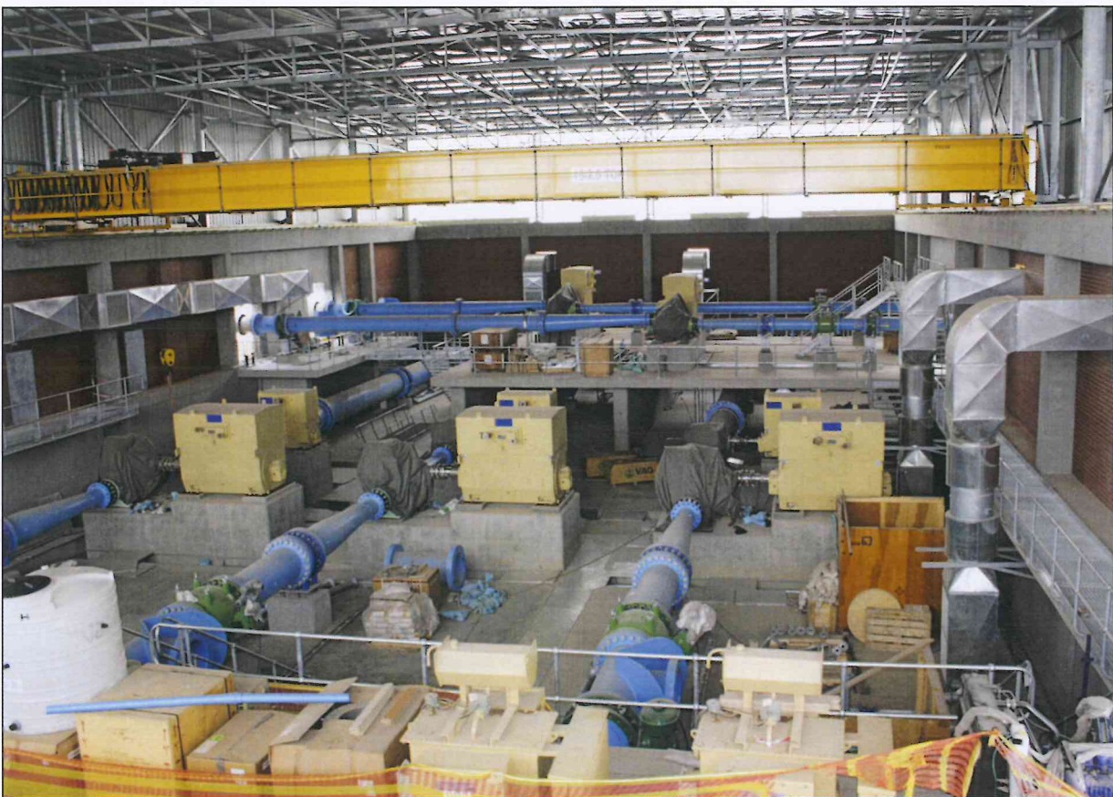
The new combined pump station for reversing the flow in the Association's pipeline and future supply to the Olifantspoort Purification Works of Lepelle Northern Water.
