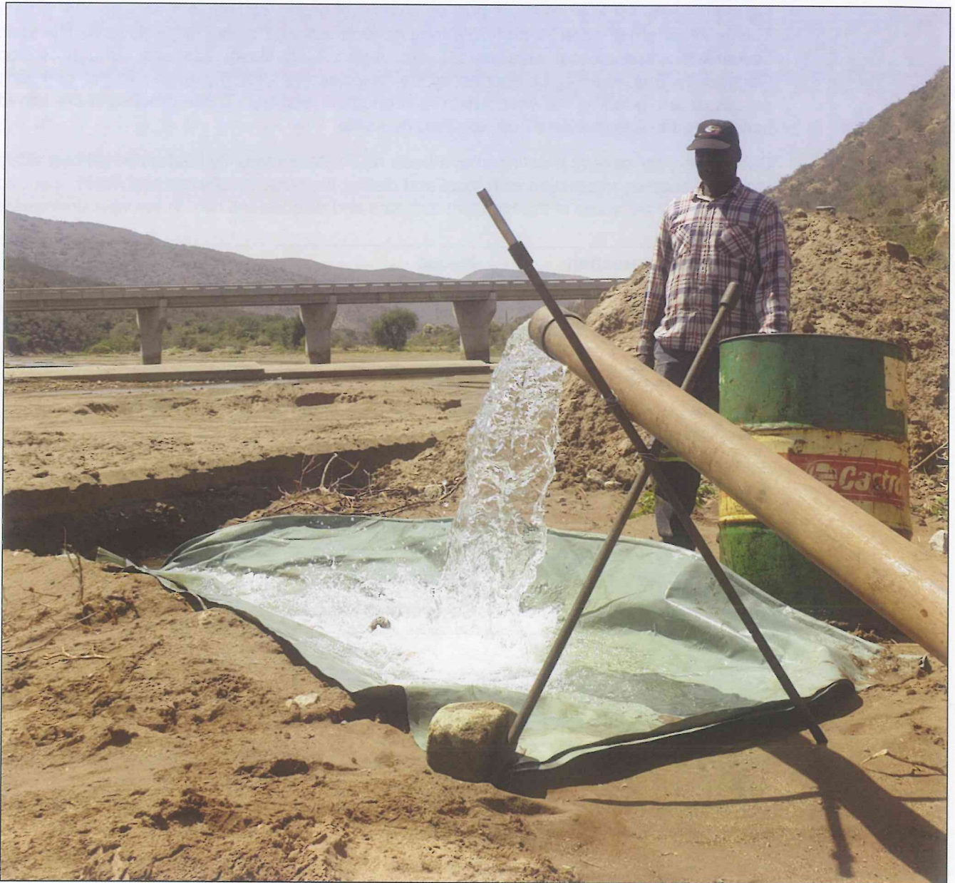
A new borehole inside the Alluvium upstream from the weir being tested.
