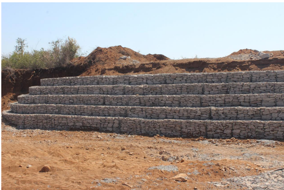
Photo 9: Clearance of vegetation found at the gabion embankment
