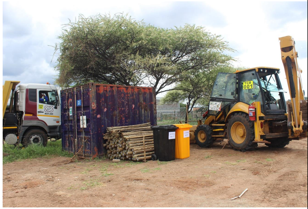
Photo 39: Waste bins along SE2 pipeline route
