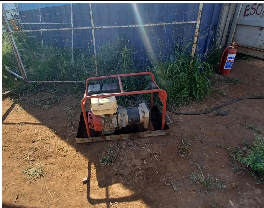
Photo 26: Drip trays under machinery
