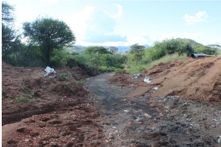
Photo 23: Soil stored in the drainageline and sandbags washed away
