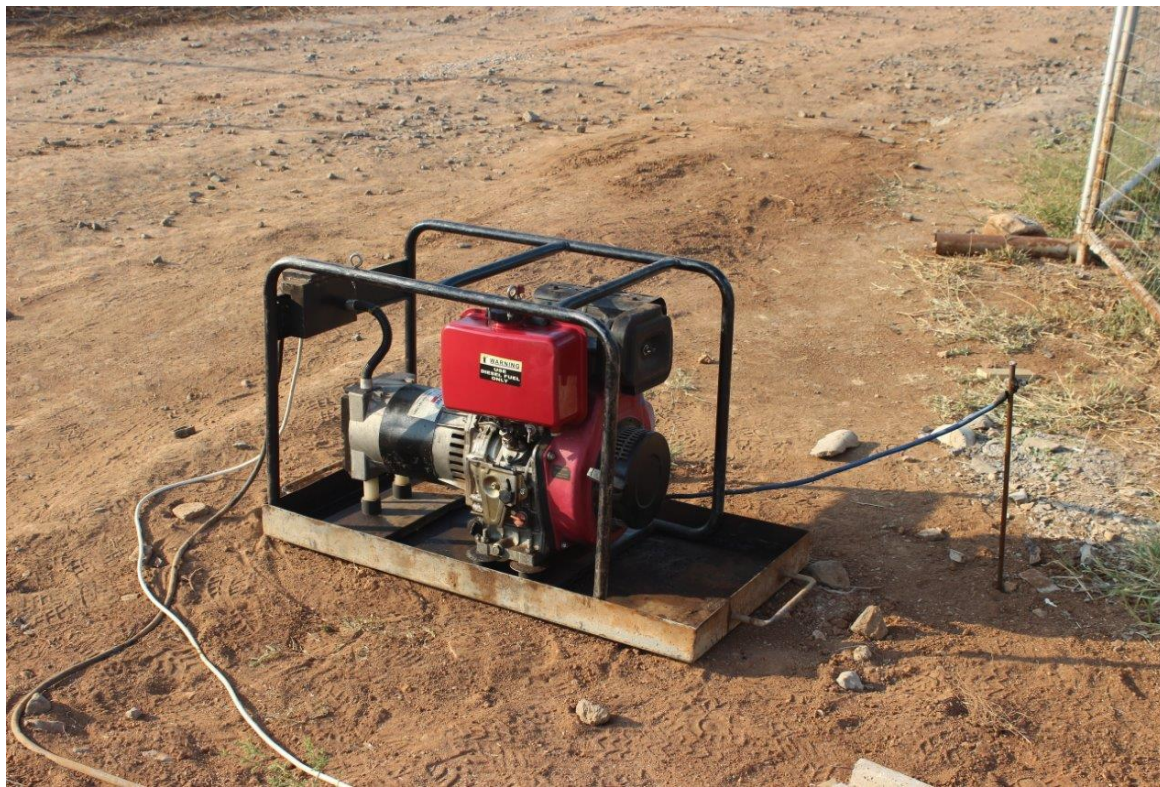
Photo 25: Drip trays under machinery not in use.
