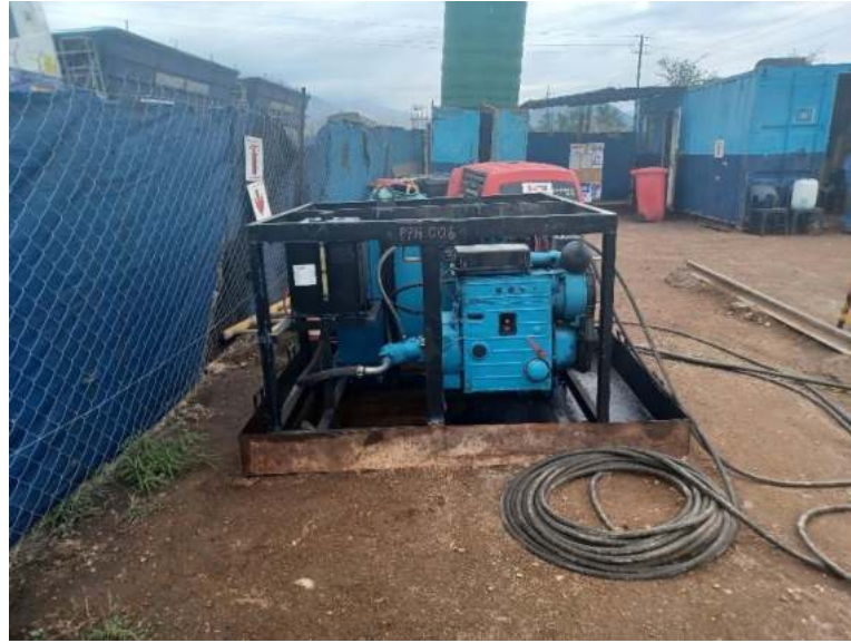
Photo 26: Drip trays under machinery not in use.
