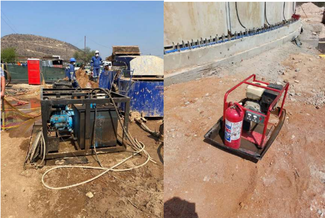
Photo 34: Drip trays used on site
