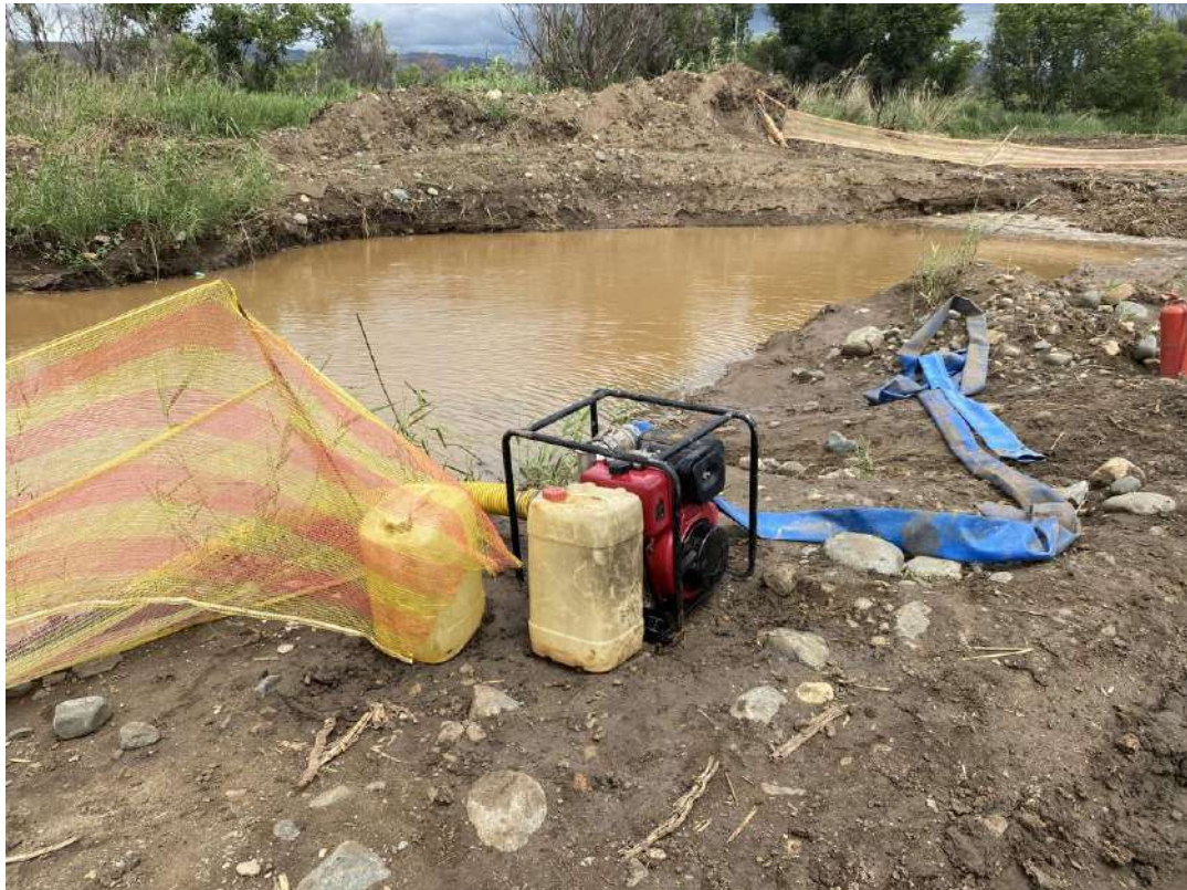
Photo 34: No drip trays found under machinery on site
