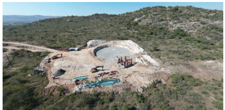
Phase 2 of the SE2 Project kicked off in July 2022 and will be completed in Q2 of 2025.
