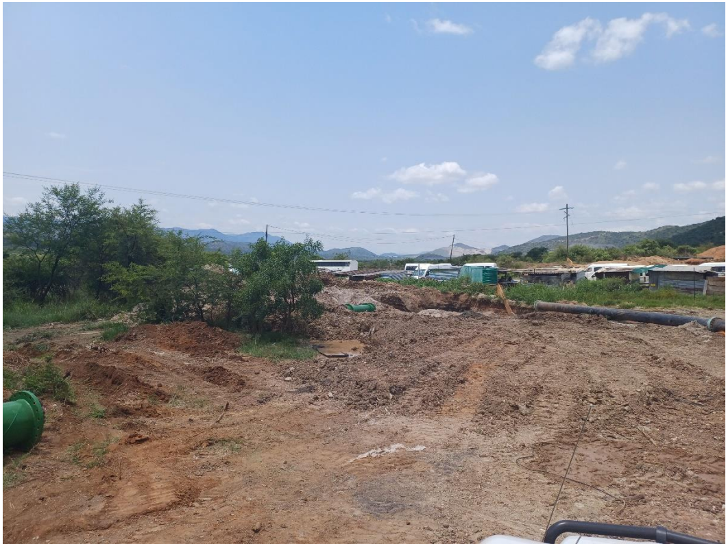
No Ablutions along Pipeline Route
