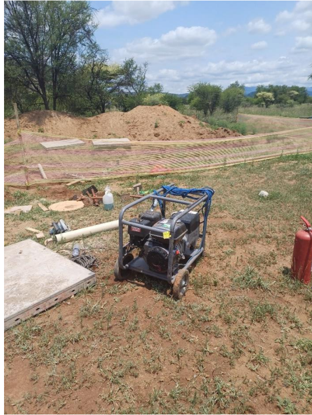
Photo 34: No drip trays found under machinery on site
