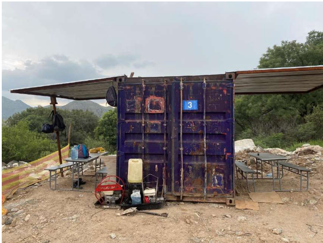
Photo 34: Drip trays found under machinery on site
